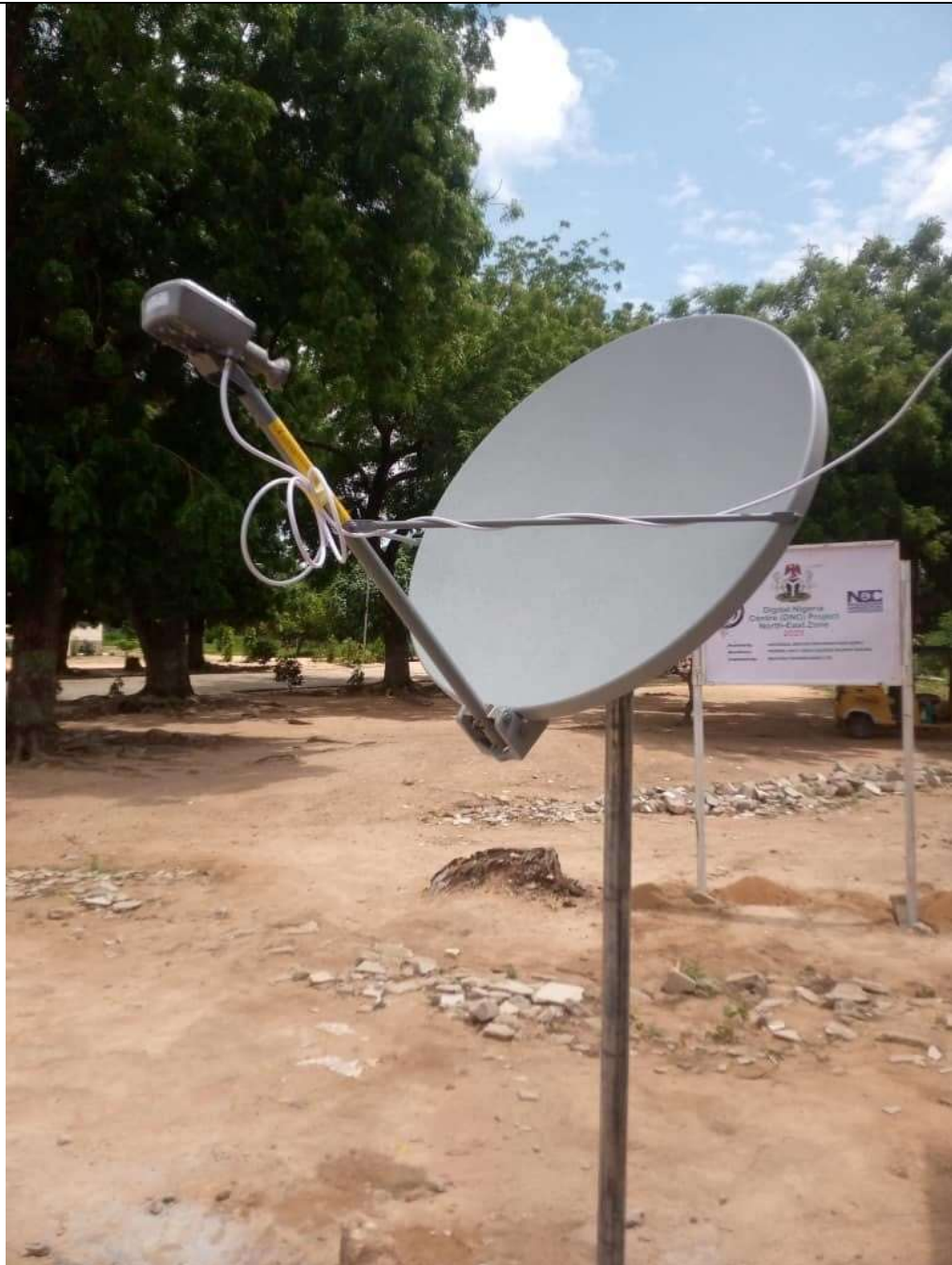
Installed VSAT Equipment
