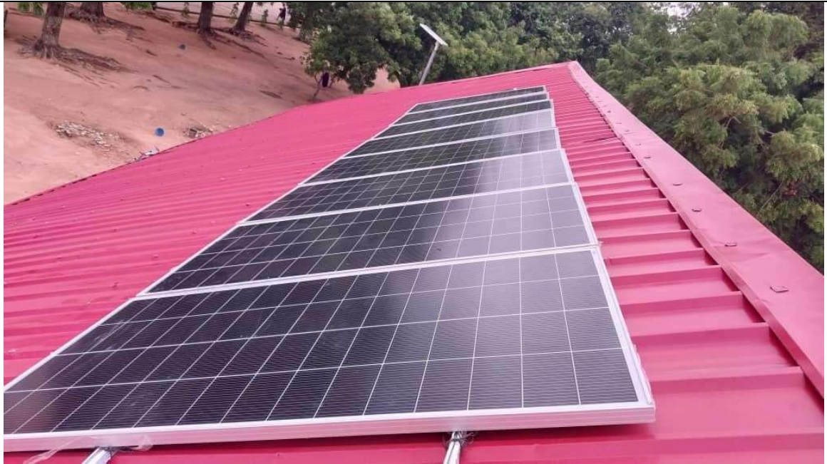
Exterior View of the ICT Building with Roof-Mounted Solar Panels
