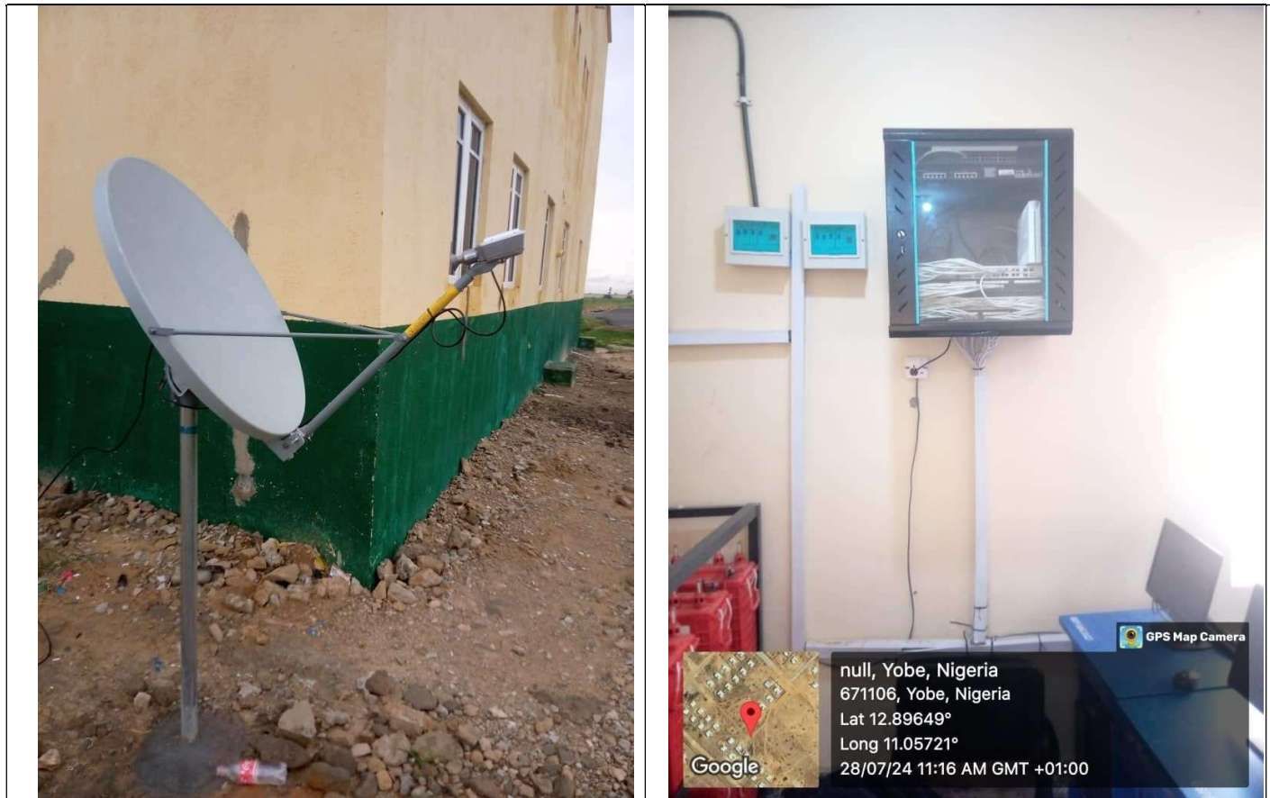
Installed VSAT Equipment and Wall-Mounted Network Rack
