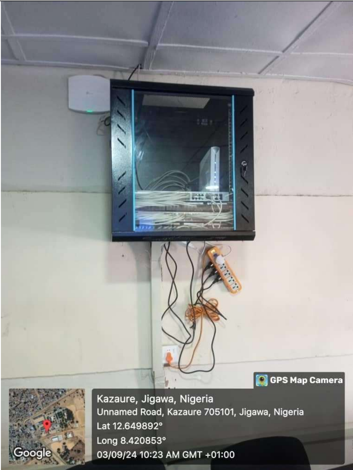
INSTALLED NETWORK RACK, ROUTERS & SWITCHES
