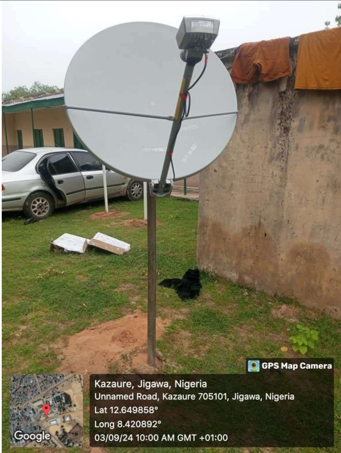
INSTALLED VSAT EQUIPMENT
