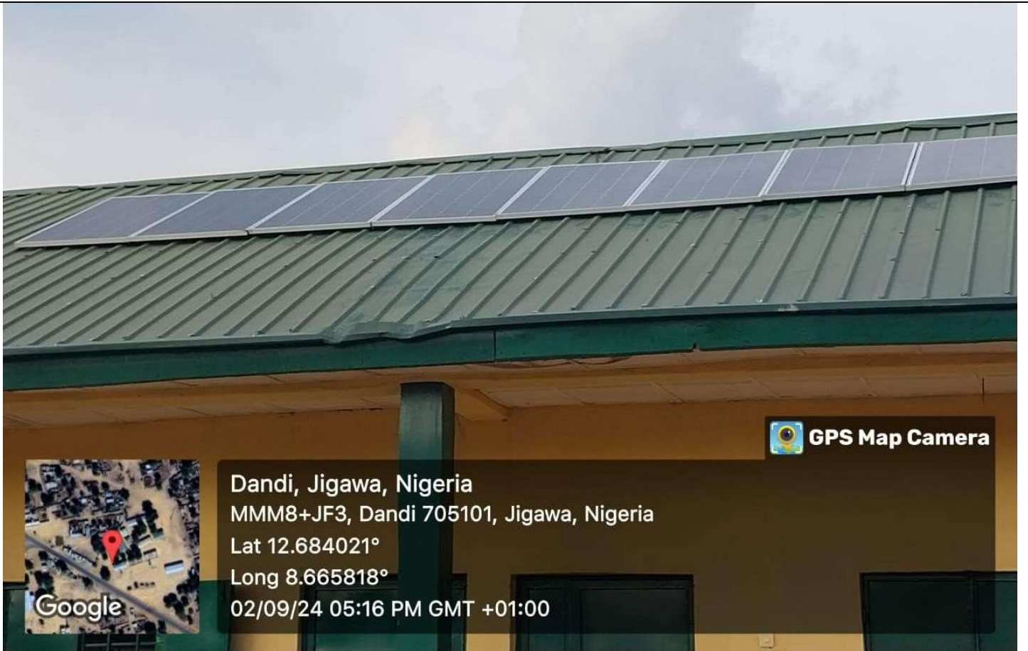
INSTALLED ROOF-MOUNTED SOLAR PANELS
