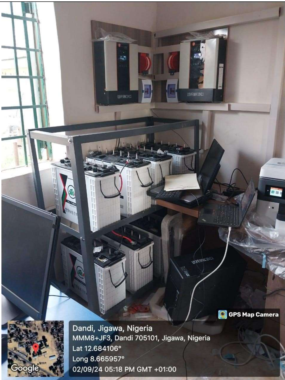
INSTALLED INVERTER SYSTEM AND BATTERIES
