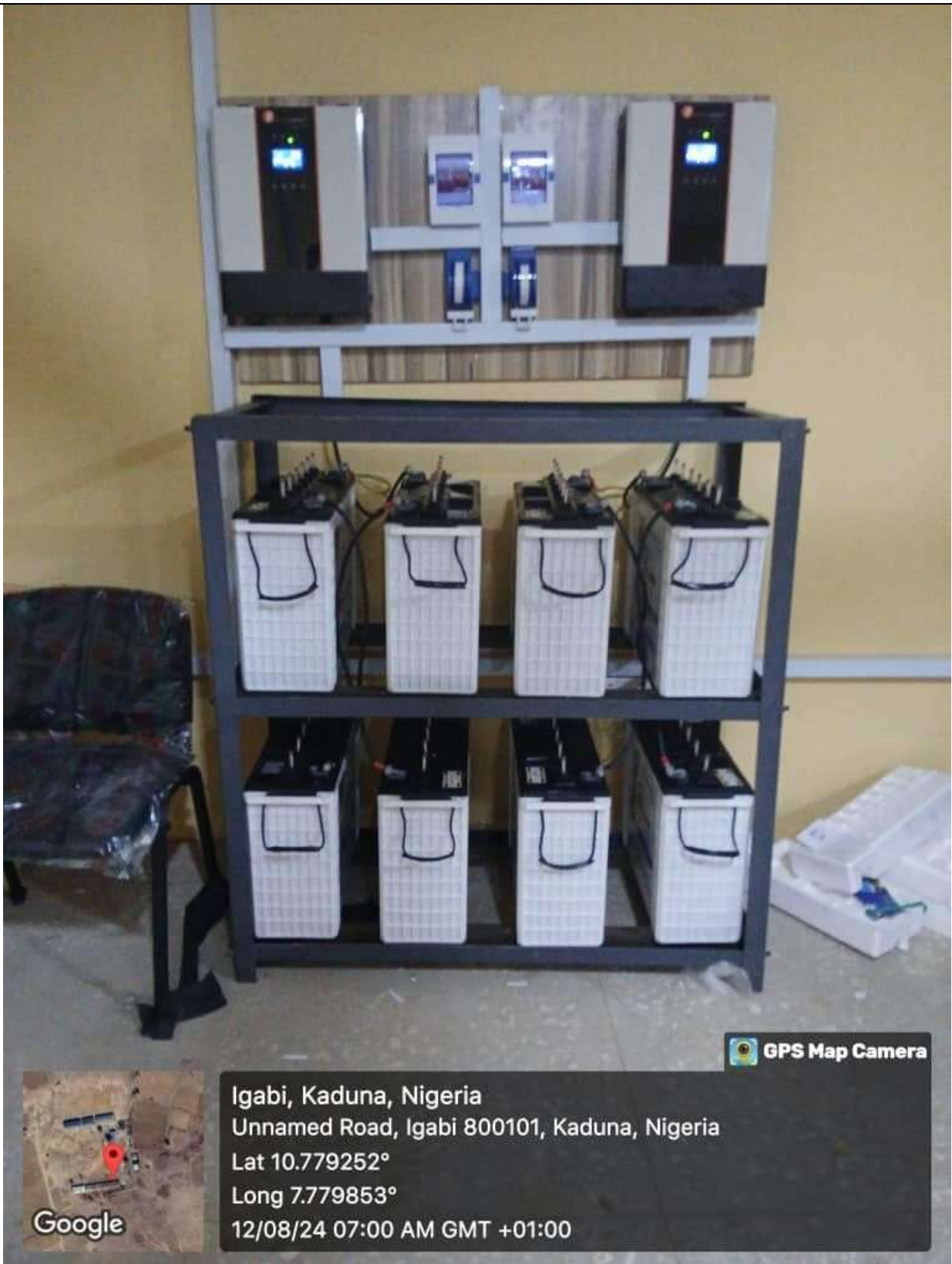
INSTALLED INVERTER SYSTEM AND BATTERIES
