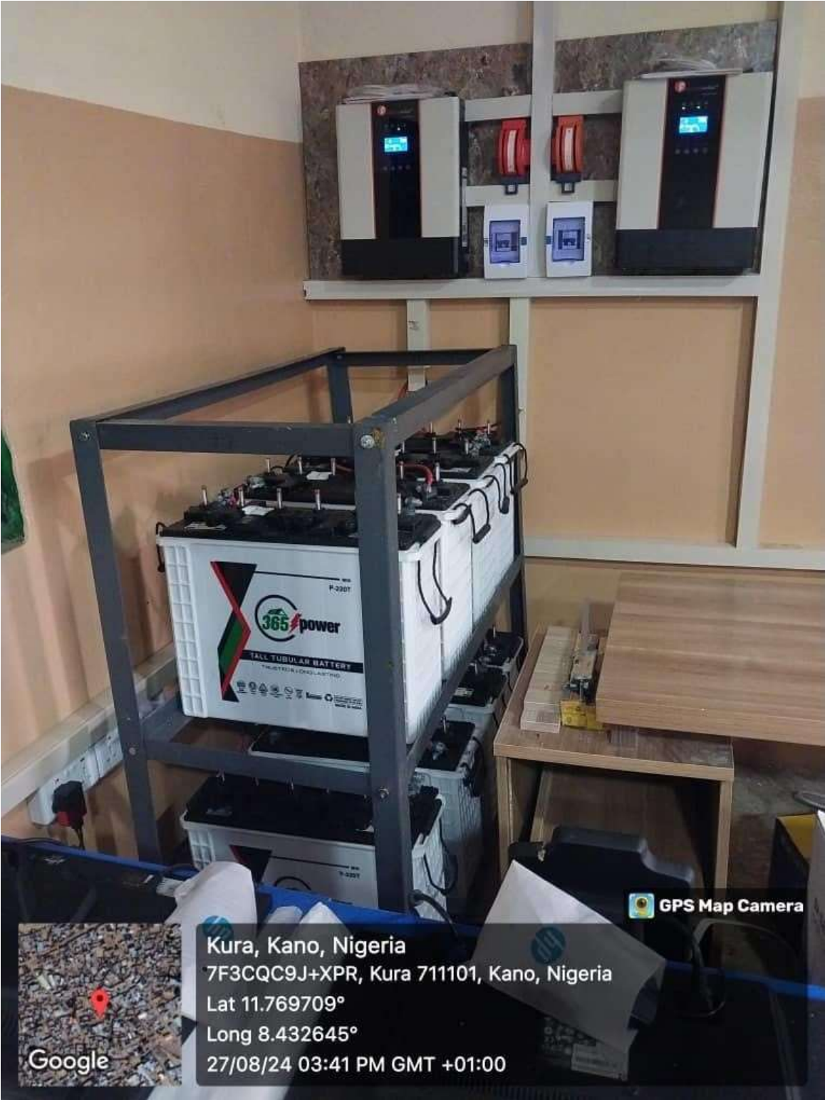
INVERTER SYSTEM AND BATTERIES
