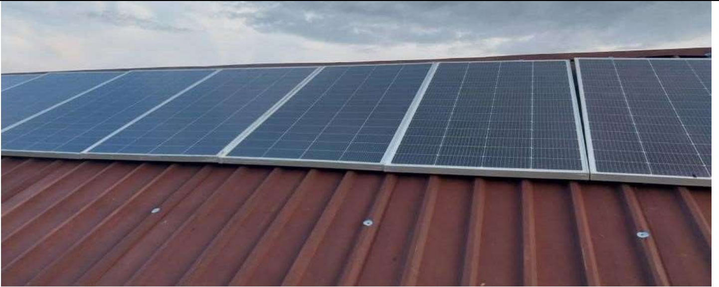
SCHOOL SIGNAGE AND ROOF-MOUNTED SOLAR PANELS
