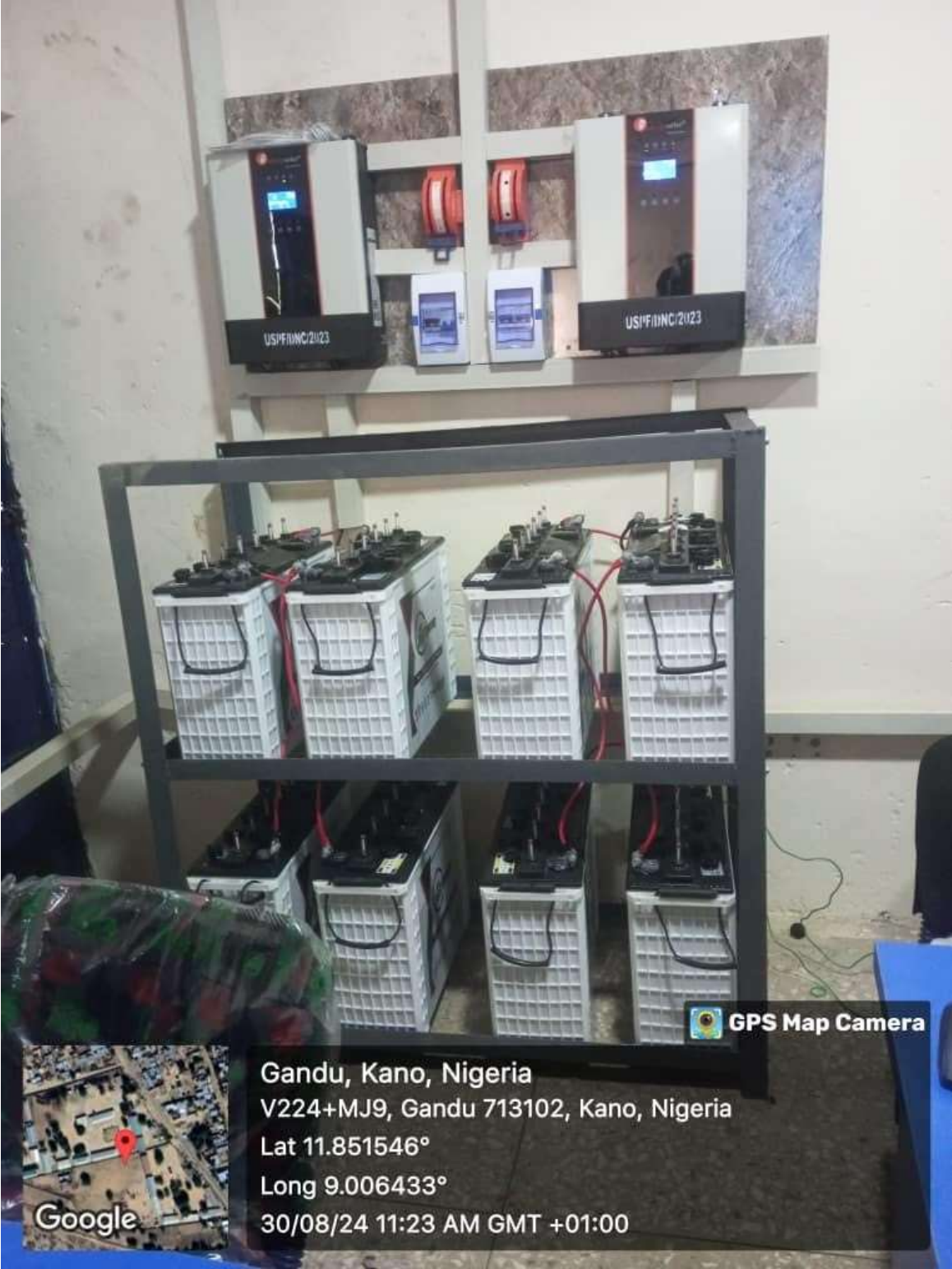
INSTALLED INVERTER AND BATTERIES
