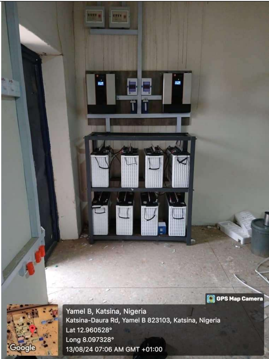
INSTALLED INVERTERS AND BATTERIES
