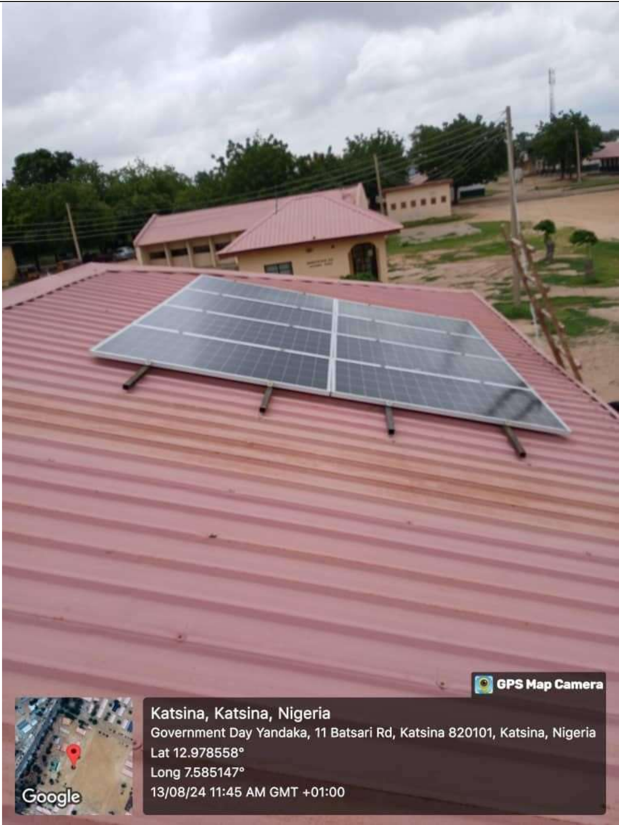
ROOF-MOUNTED SOLAR PANELS
