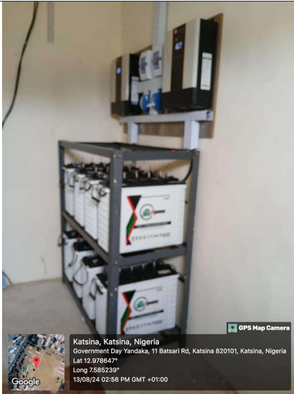
INSTALLED INVERTERS AND BATTERIES
