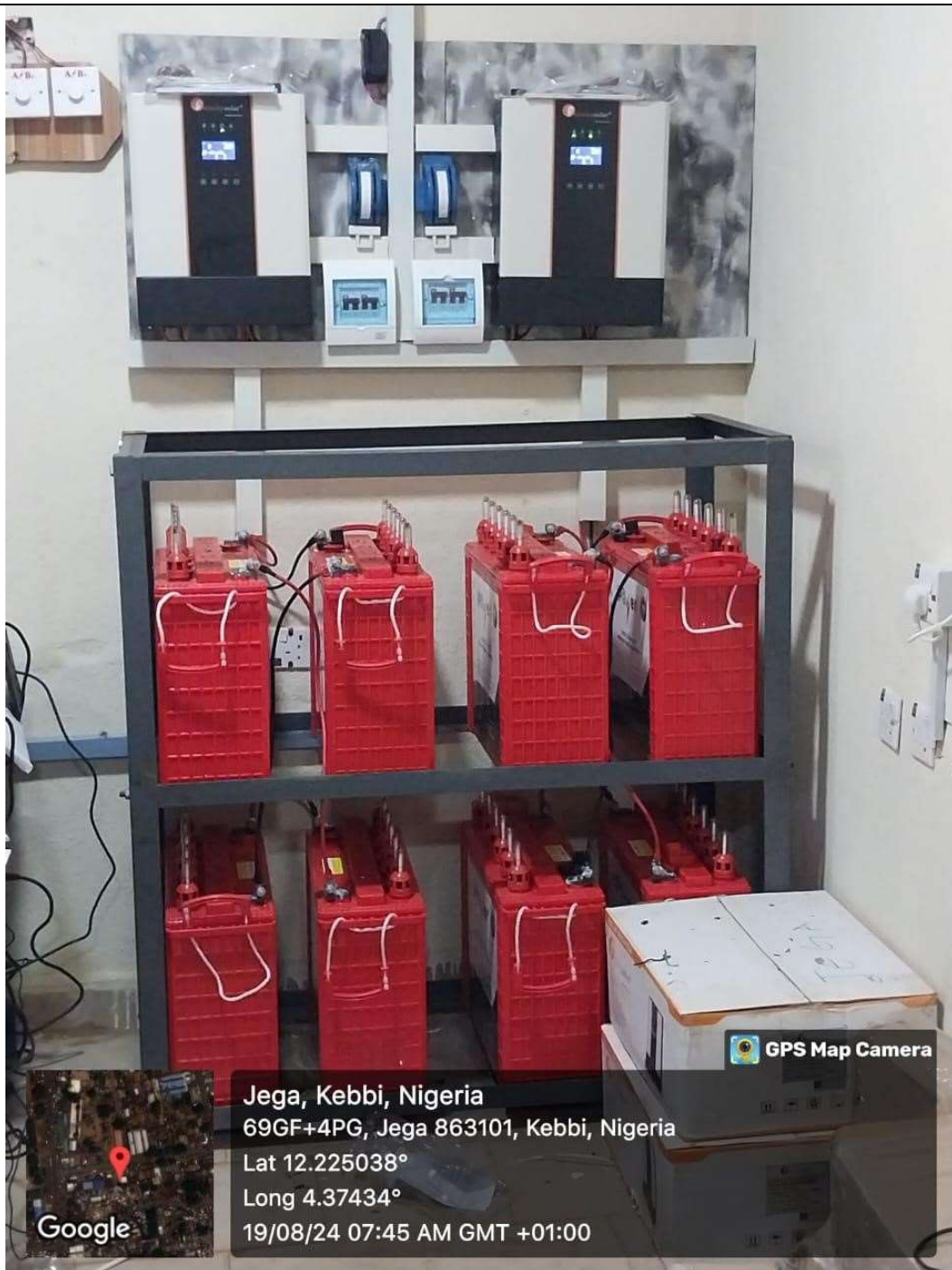
INSTALLED INVERTERS AND BATTERIES
