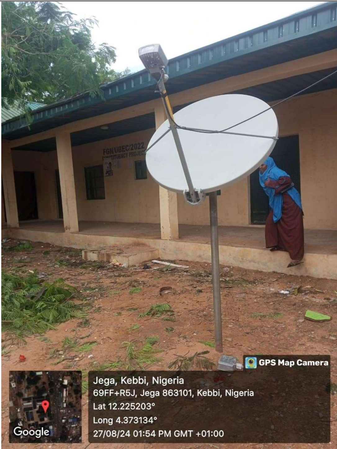
INSTALLED VSAT EQUIPMENT
