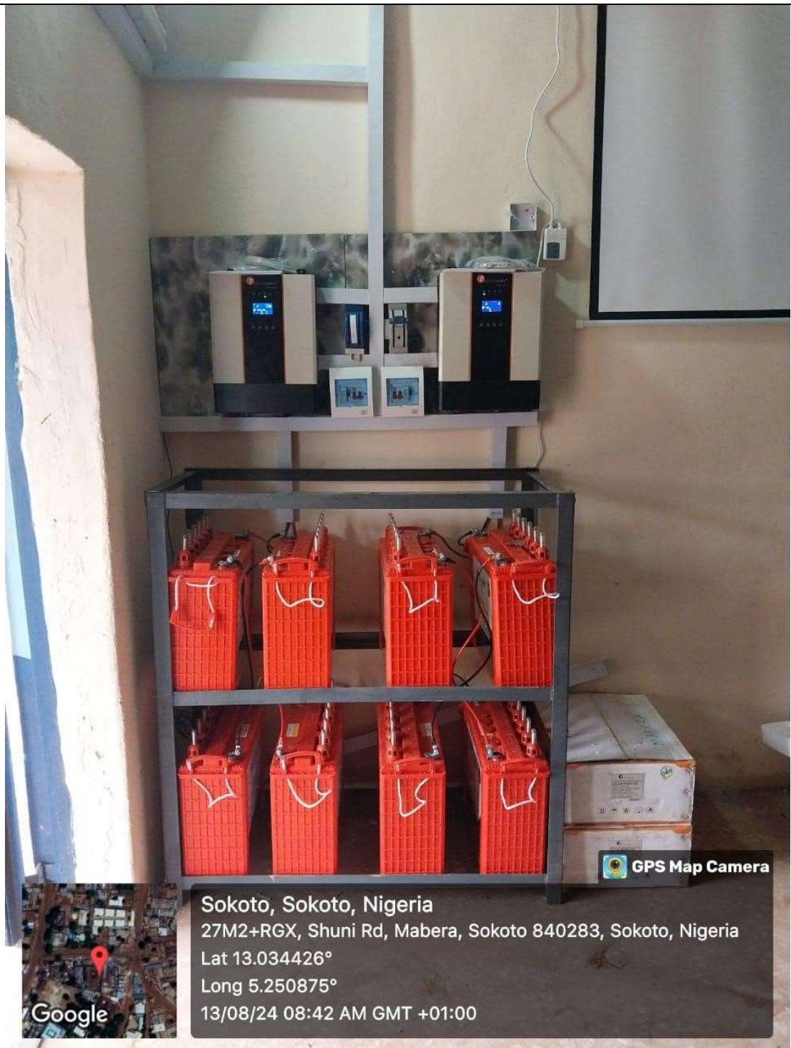
INSTALLED INVERTERS AND BATTERIES
