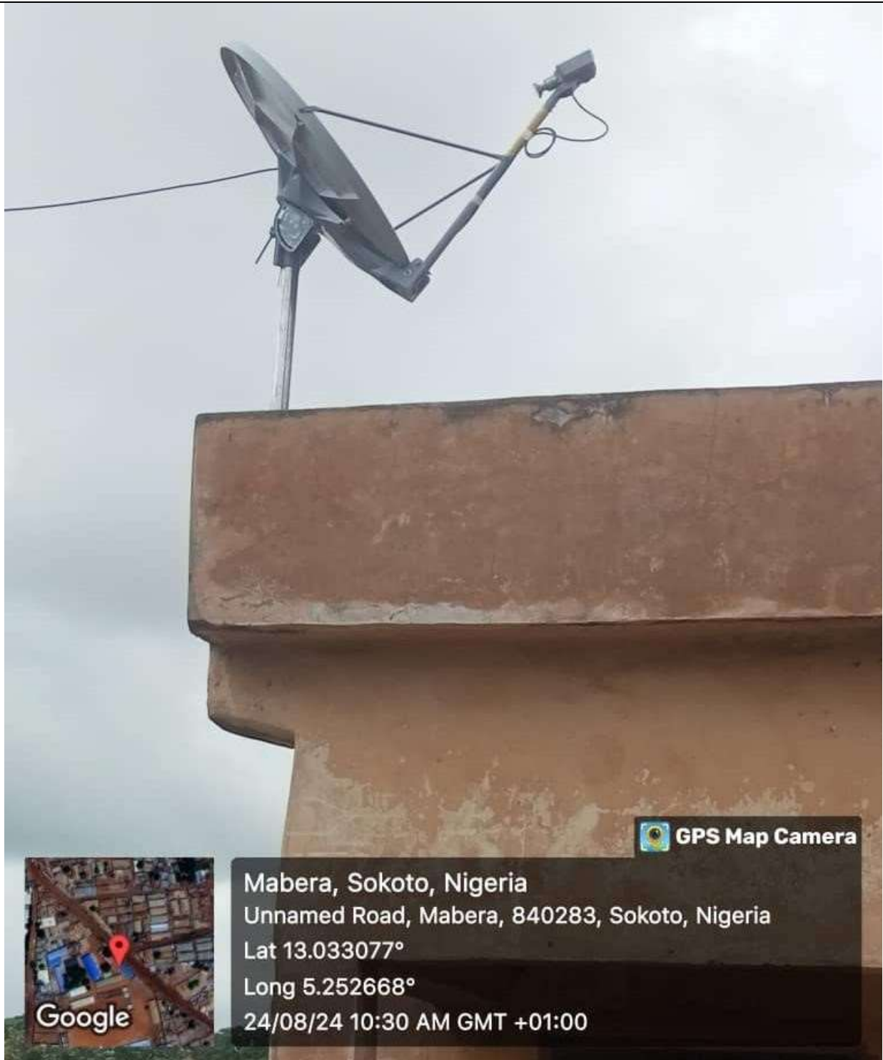
INSTALLED VSAT EQUIPMENT
